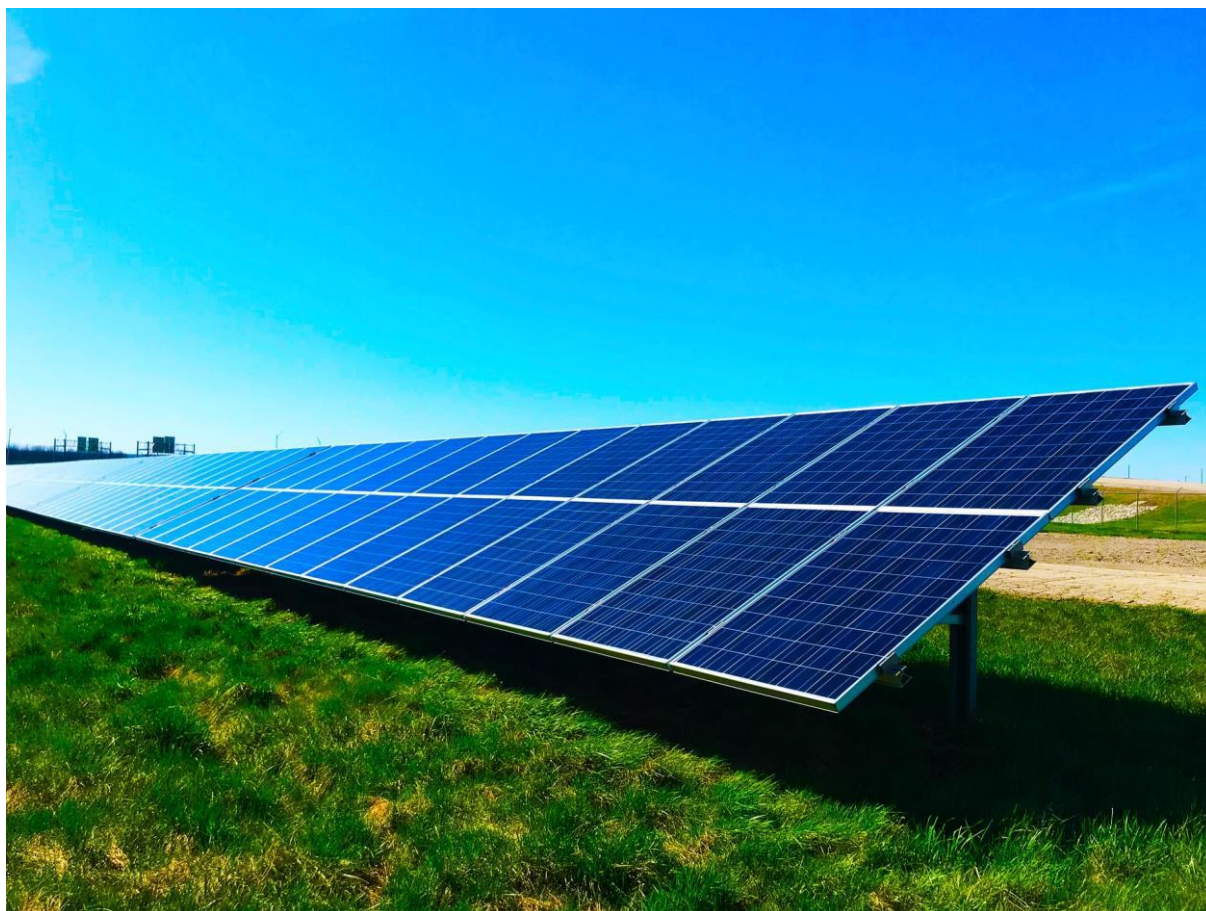
Fig. 11. Example of a photovoltaic installation
