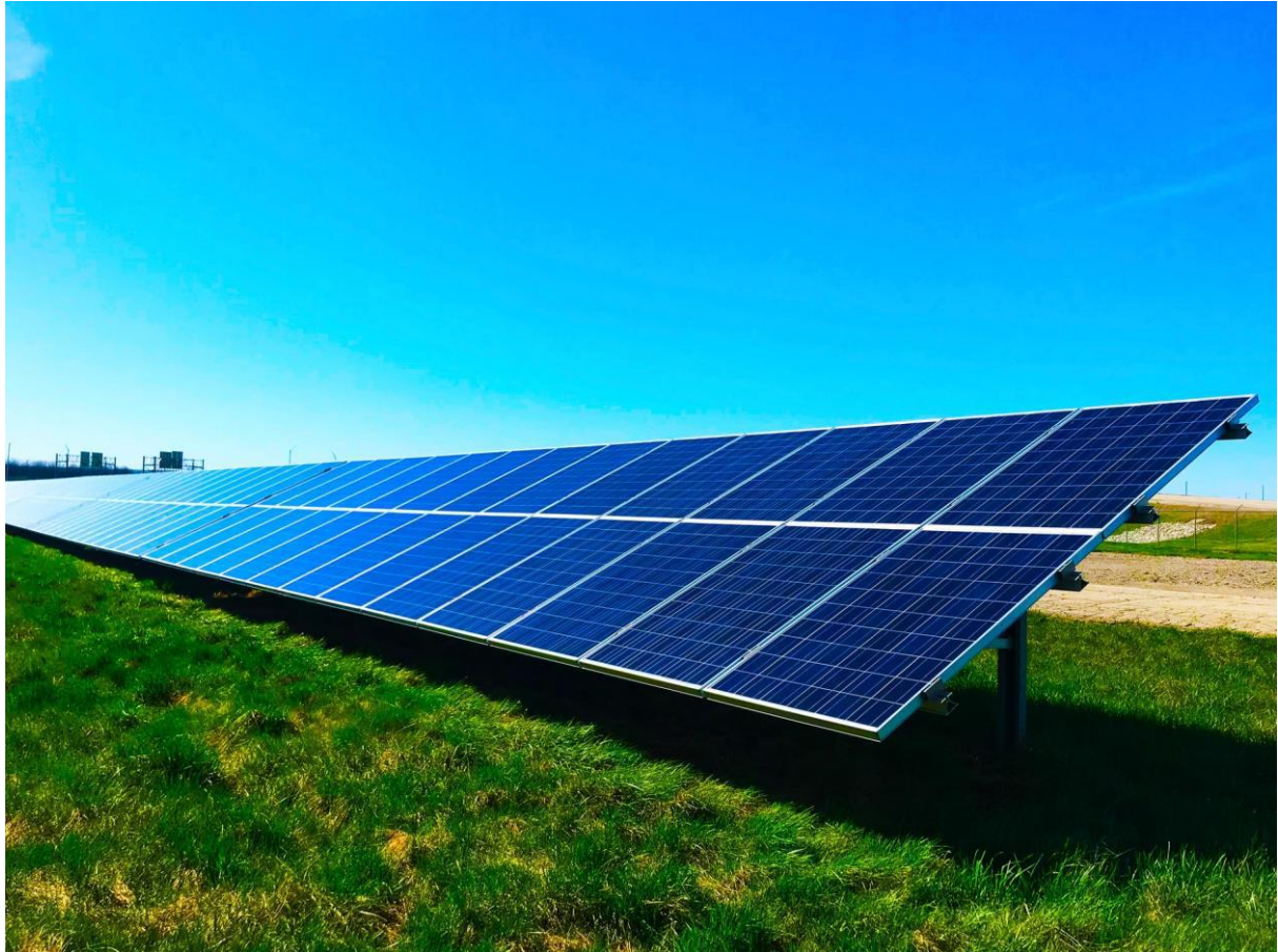
Fig. 11. Example of a photovoltaic installation
