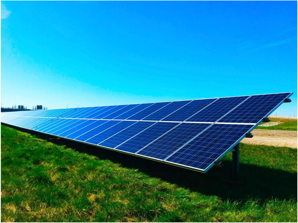
Fig. 11. Example of a photovoltaic installation
