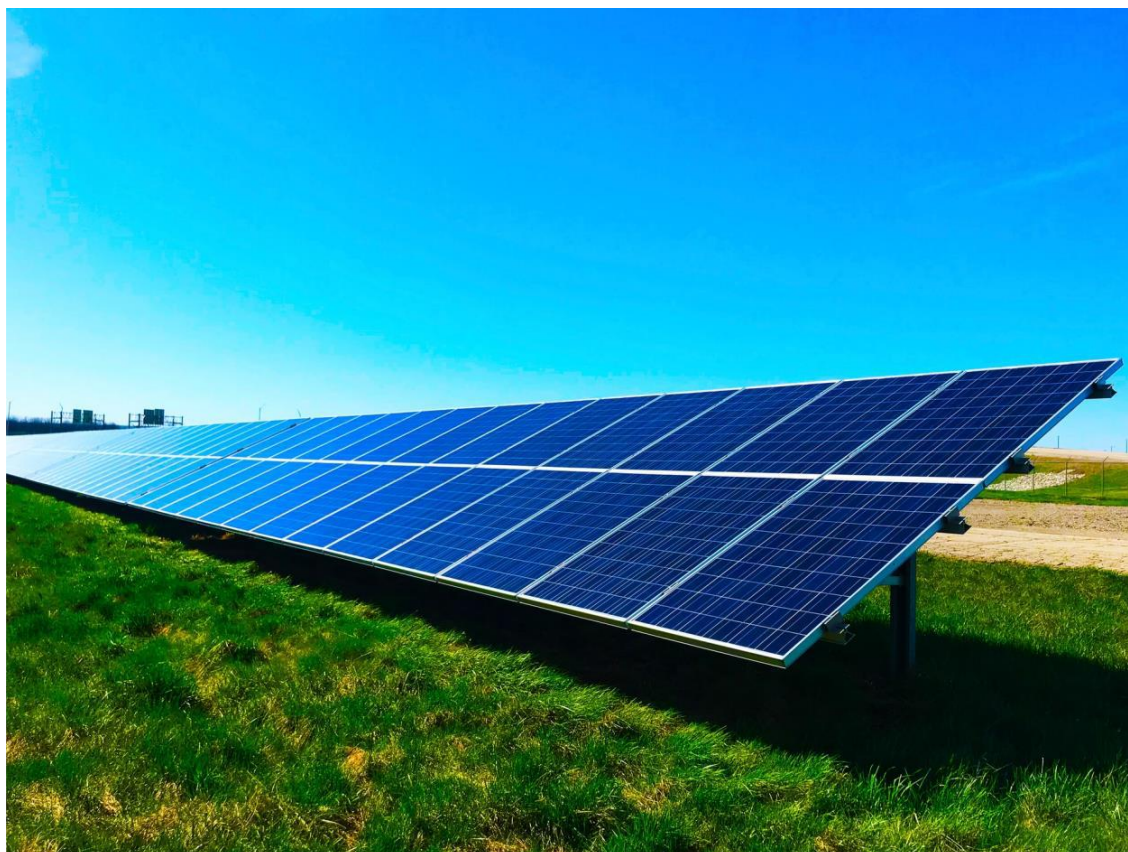
Fig. 11. Example of a photovoltaic installation
