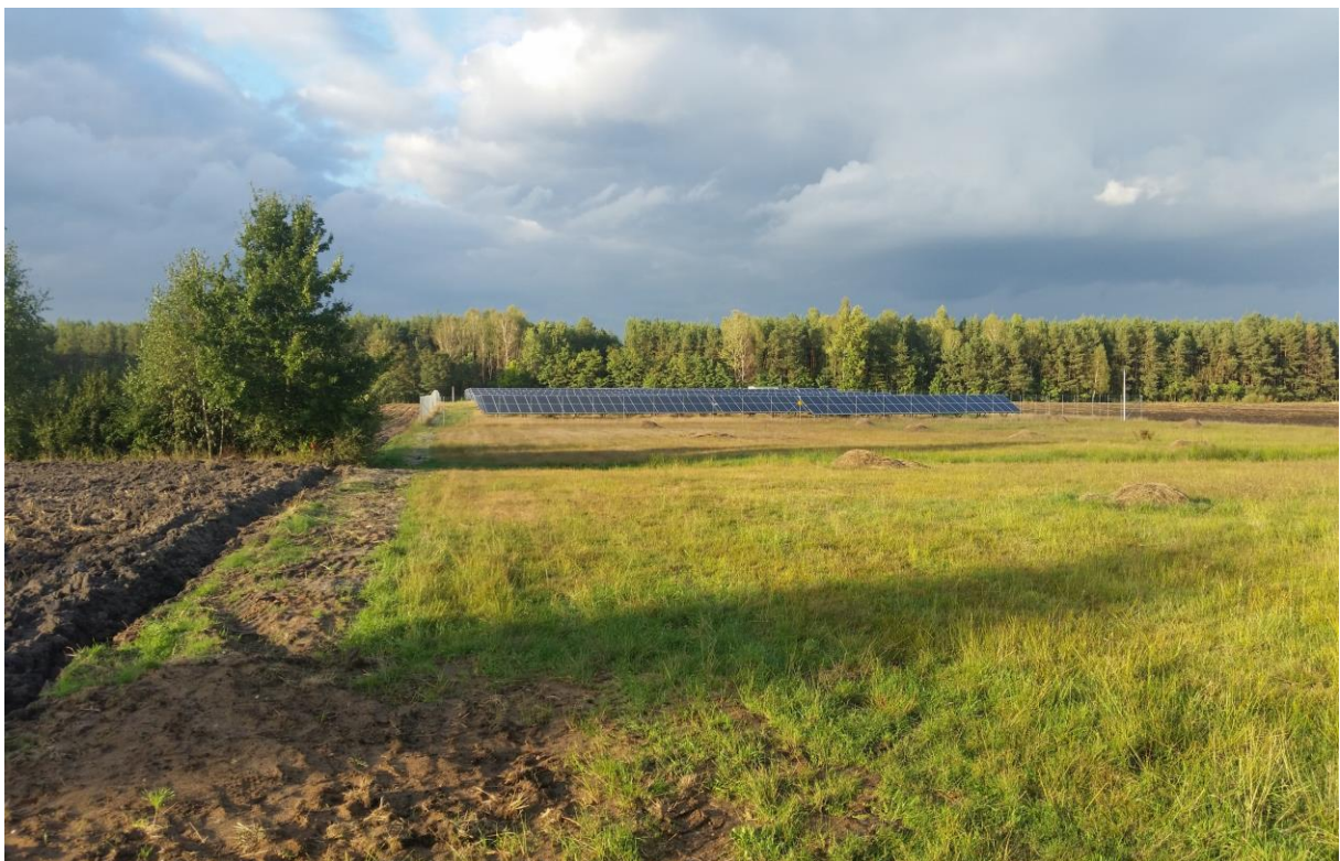
Z-5.2 Photographs of an example photovoltaic system (solar power station) built in Poland.
